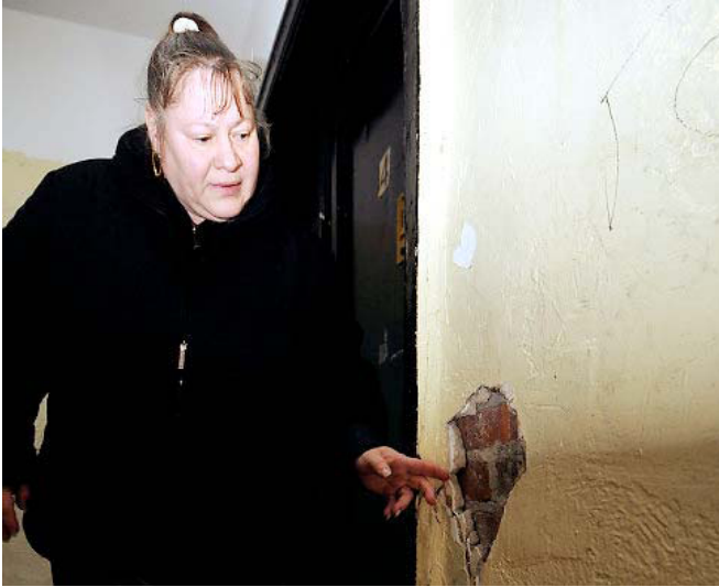
Harbus for News Gladys Gonzalez points out cracked hallway at 1553 Bryant Ave., where she lives.
